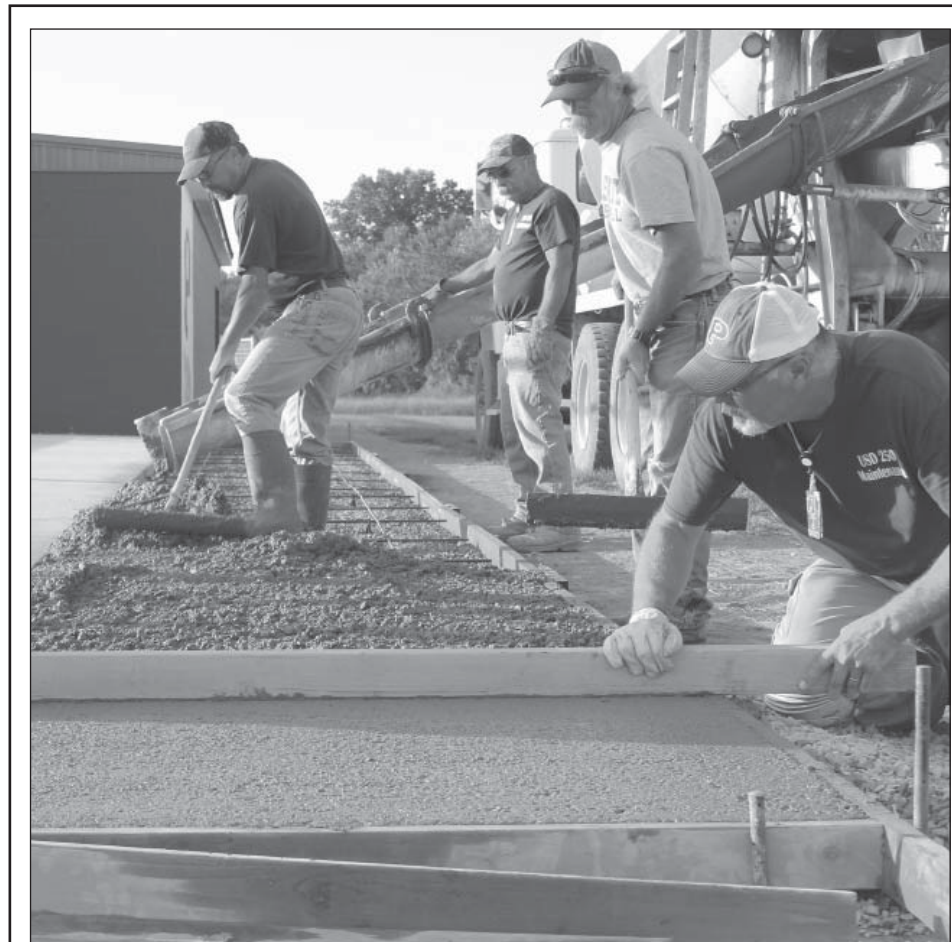
Finishing one of the last sidewalk segments, workers smooth out concrete on the softball complex. The team will be play its first home game this spring. PHOTO BY MIRANDA MOORE
